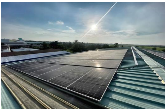
Mitsubishi G-Star Ca Mau 100 kWp commercial rooftop • 2024
