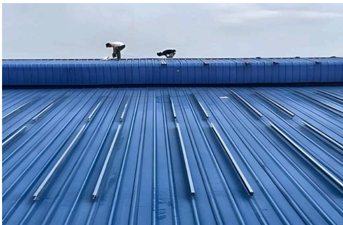
Guardianmade – Ba Ria-Vung Tau 1,000 kWp industrial rooftop • 2024
