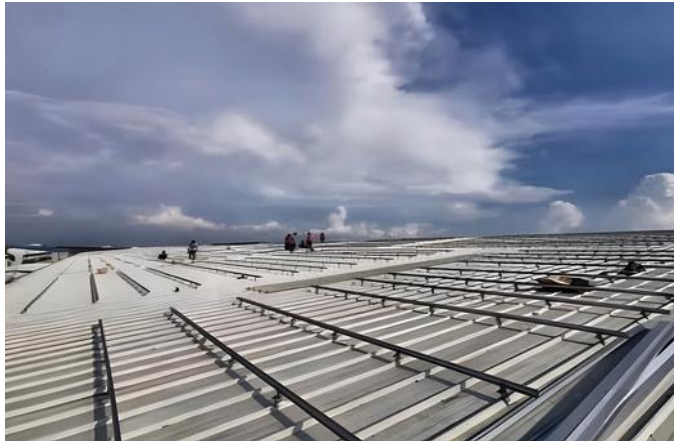
Trung Nguyen Coffee – Dak Lak 1,000 kWp industrial rooftop • 2022
