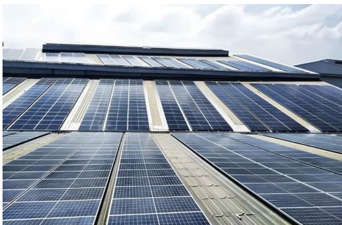
Hung Phuoc Food JSC – Can Tho 7,000 kWp industrial rooftop · 2020
