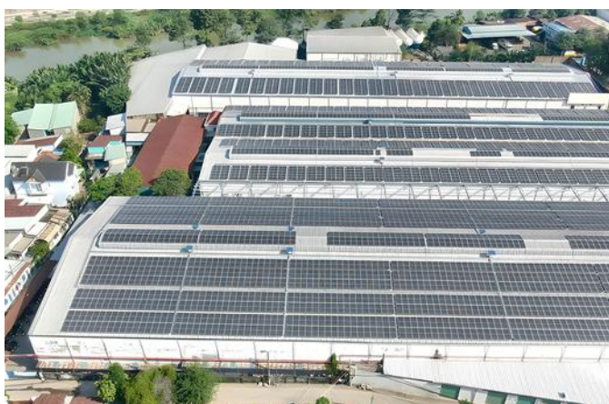
Hung Thinh Vina Garment – Thu Duc 3,200 kWp industrial rooftop · 2020
