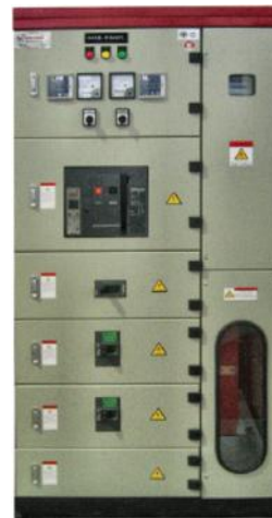
MCCB distribution board ទូរចែកចាយ MCCB
