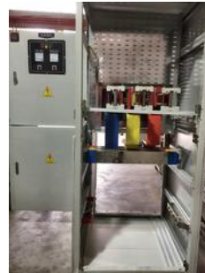
MV switchgear panel
