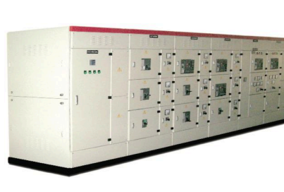
Main switchboards ទូមេ (MSB)
